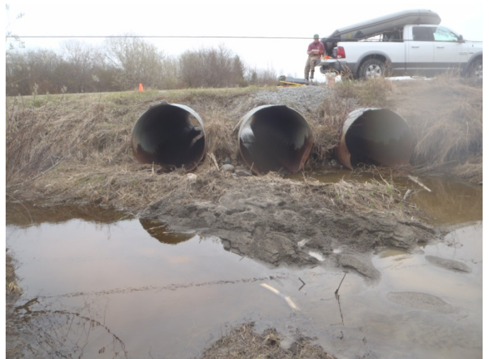
Photo 16: Facing culverts at Highway 600 road crossing, downstream at LOS-1A, on Loslo Creek. AMEC field staff taking field notes.
