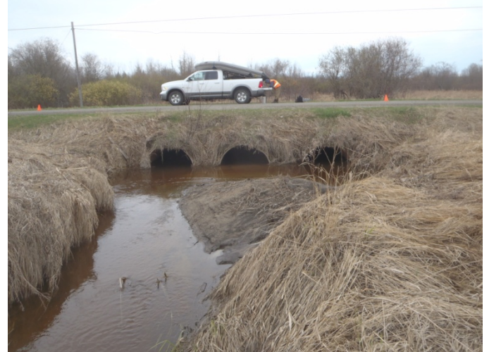
Photo 24: Culverts at Highway 600 road crossing, facing upstream, at WES-LOC F, on West Creek.
