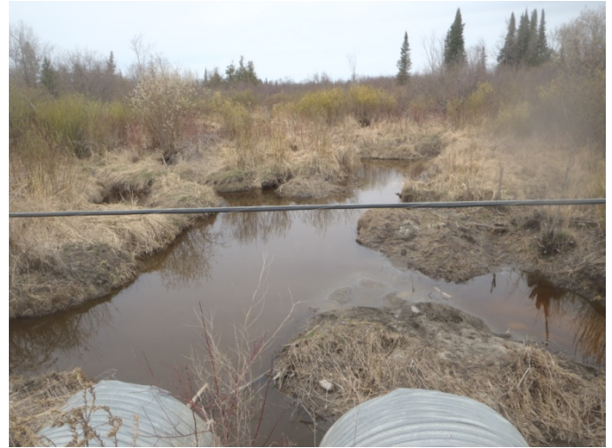
Photo 14: At Highway 600 road crossing, facing northeast, upstream at LOS-1A, on Loslo Creek.
